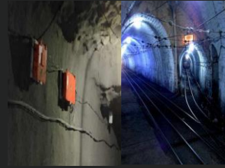
Underground sensing equipment connection
