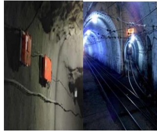
Underground sensing equipment connection
