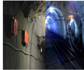
Underground sensing equipment connection
